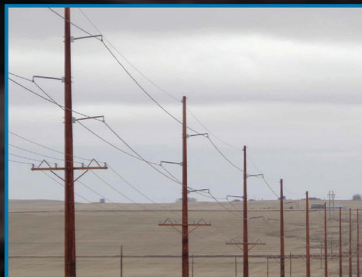
Distribution & Transmission Poles
